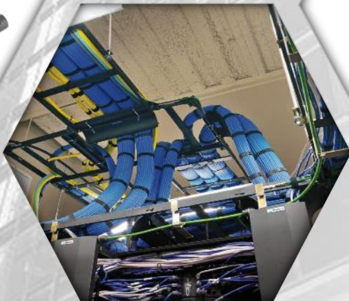
Cabling and Cable Management
